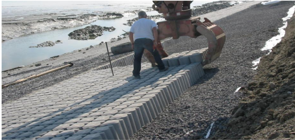
Figure 3.1 Concrete columns. The photo also shows the granular filter and a geotextile.
